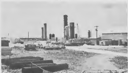
RAPIDLY TAKING shape is the industrial profile of the Antilles Chemical Company at Baredera. The towers and drums are the gas cleanup area. At right is the company's warehouse.
